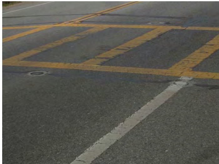
Figure 1. In-pavement lights covered by striping.
